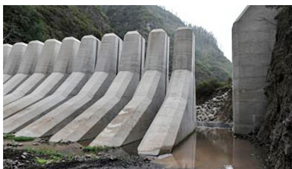
Fig. 13: Weir located on the Santa Luzia stream (Funchal) (Source: Authors)
